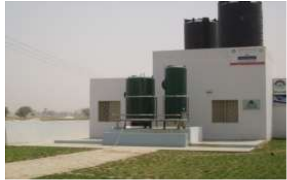
Fig. 18 Water filtration plant in Miani Mallah Source: Photograph by the Authors, 2011
