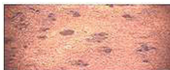
Defective Base Metal.
