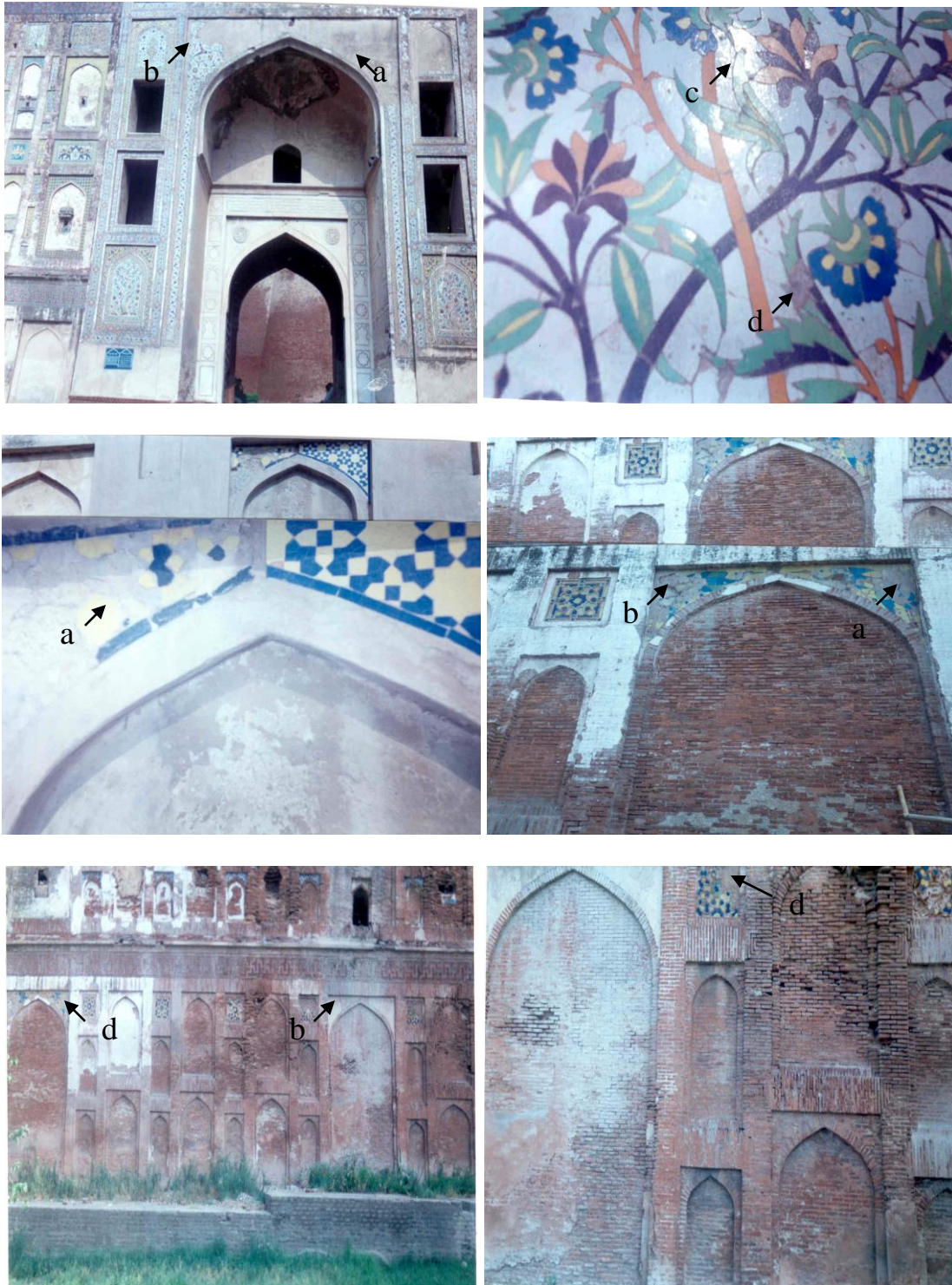
Plate 1: Extent of decay at various sampling sites of Picture walls at Lahore Fort a: peeling off, b: discoloration, c: staining, d: cracking
